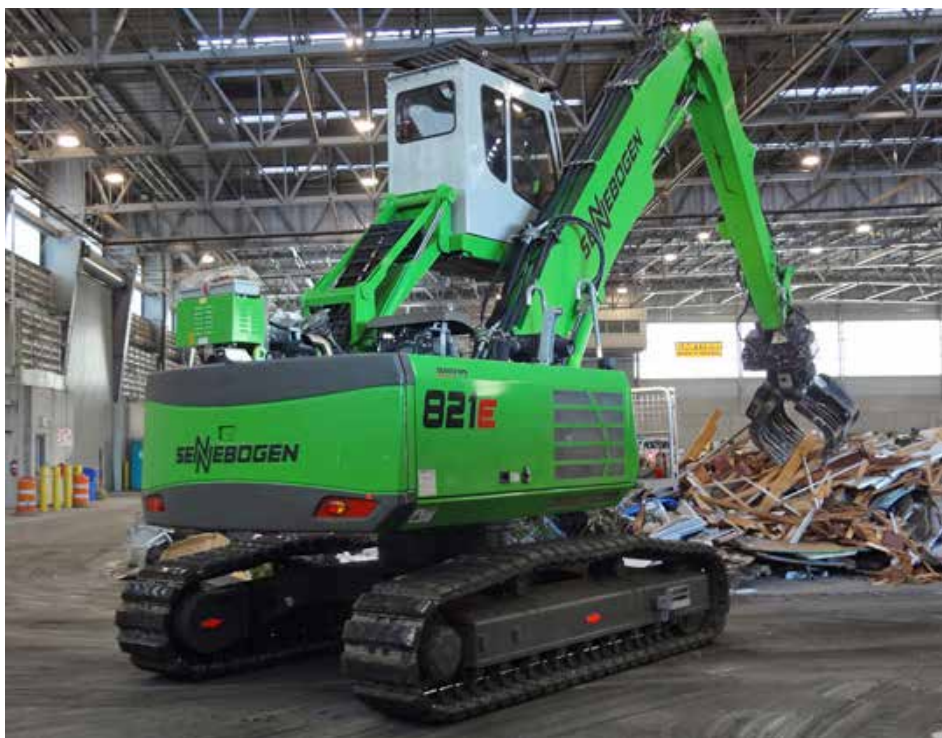
The 821 R-HD equipped with rubber pads and a grapple works at the LEEDS certified Tacoma Recovery & Transfer Center.
